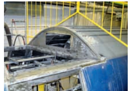
Roof cut-out for the retrofit of an air conditioning unit of a passenger car on a double-decker commuter train of the S-Bahn Zurich
